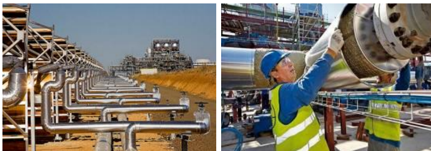
Figure 71 Solar field piping; one header pipe transports the cold oil to collector, the second header pipe transports the heated oil back to the power block; (source: Estela Solar, 2010); Assembly of the piping (BilfingerBerger, 2010)
