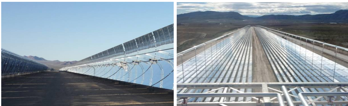
Figure 2 Line-focusing systems: Left: Parabolic trough collector: 64 MW el power plant Nevada Solar One ; dimensions: collector aperture width 5 m (Morin, 2010). Right: Linear Fresnel Collector: 1.4 MW el plant PE1 in Murcia, Spain; dimensions: Receiver height above mirror field: 7 m (Novatec, 2010)
